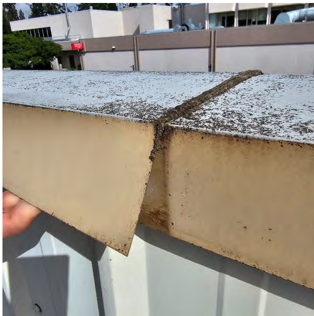
Photo 2.11: Loose parapet connection
