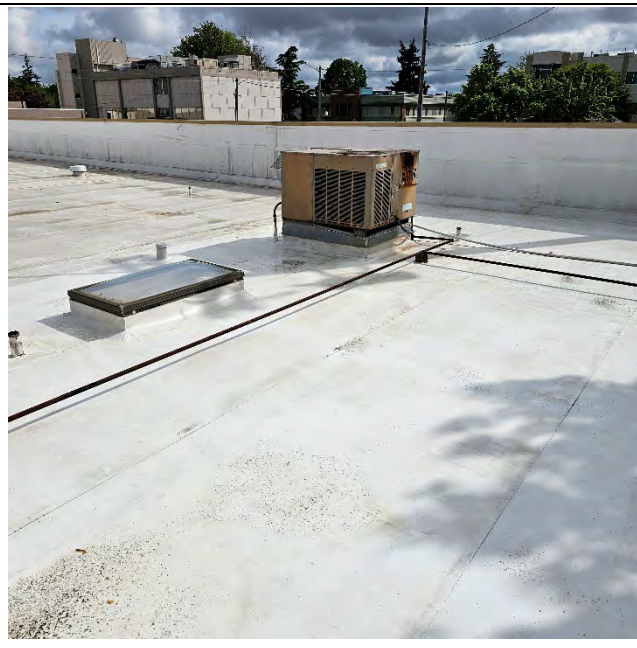
Photo 2.5: Curb mounted skylight and hvac unit
