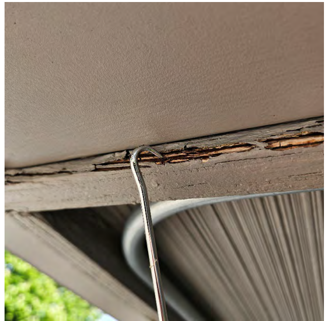
Photo 3.12: Water damaged fascia
