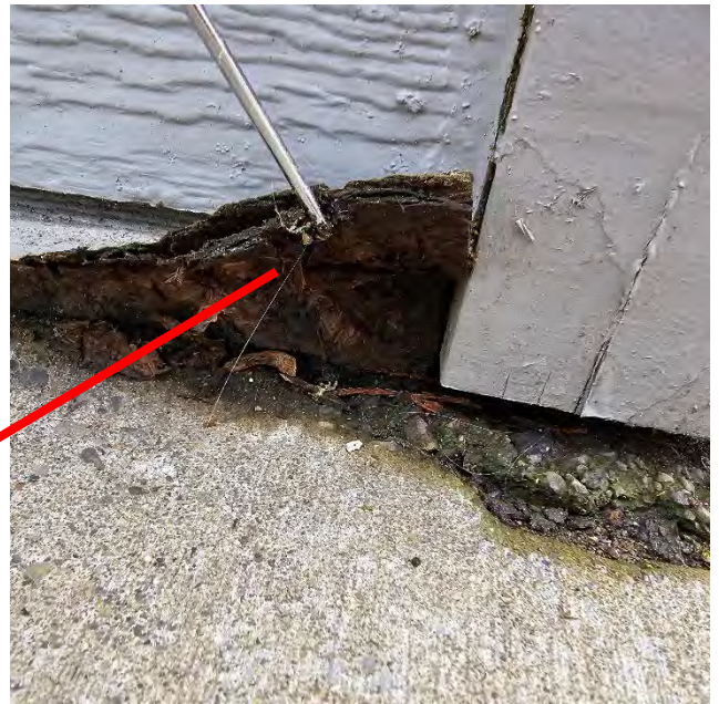
Photo 3.8: Exposed wood at transition
