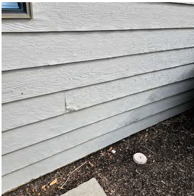
Photo 3.13: Delaminating siding at West elevation
