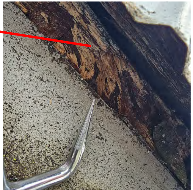
Photo 3.10: Exposed sheathing at upper edge of gutter
