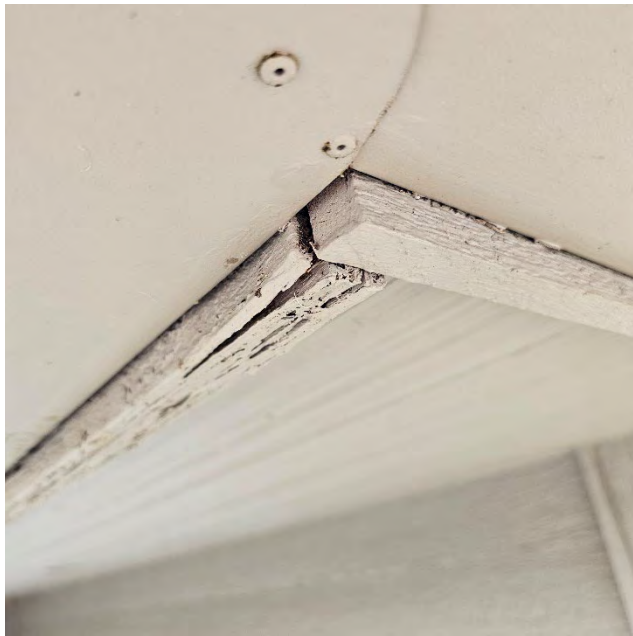
Photo 3.11: Water damaged fascia at outside corner (typ)
