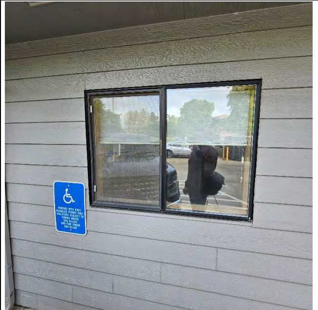
Photo 4.2: Transom window sill at entry
