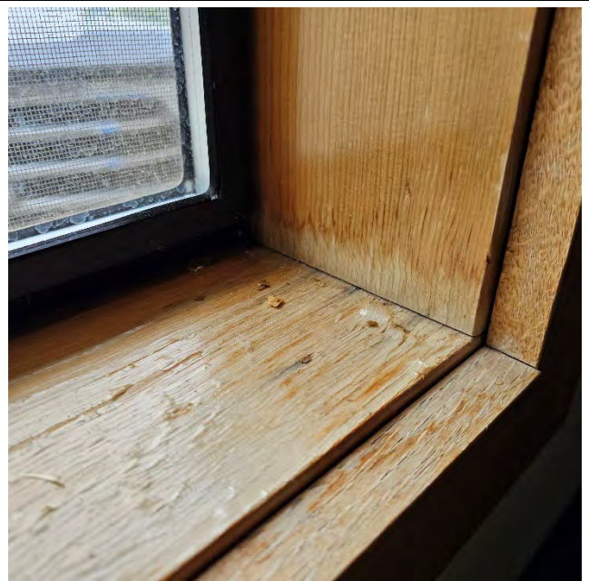
Photo 4.6: Sealant failure detail
