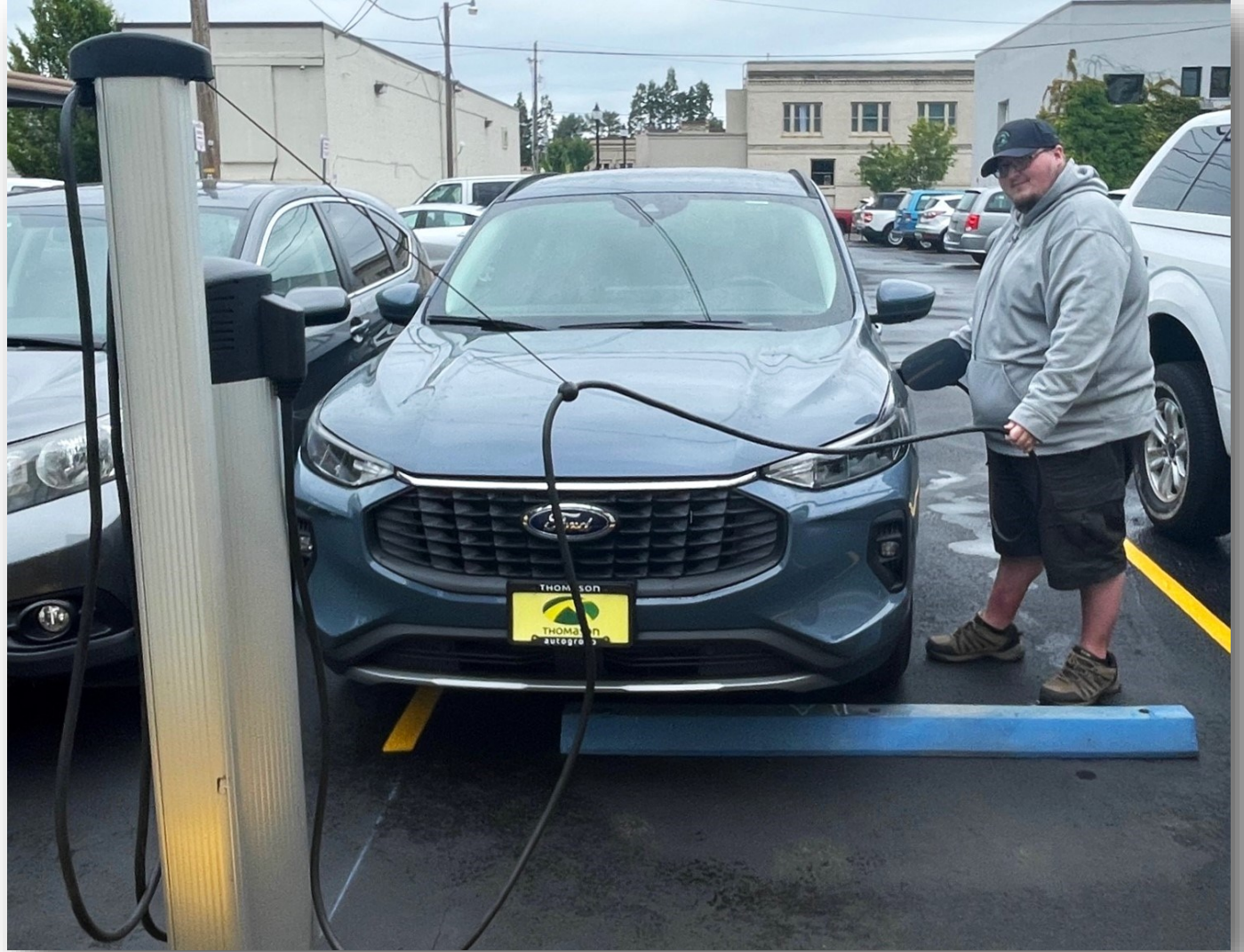
Linn County Vehicle Technician Brandon Newquist plugs in the county's new hybrid Ford Escape, using one of the new EV charging stations at the General Services fleet center next to the Courthouse Annex.
